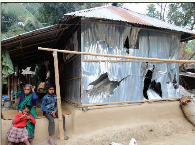
Jamaat-Shibir supporters destroyed houses of minority community people of Chapatala village of Obhaynagar upazila under Jessore district at the evening of Election Day.
