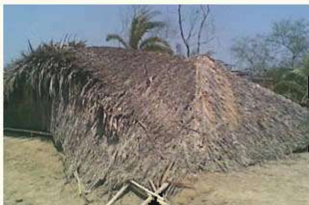
The cyclone-damaged school
