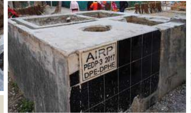
Many in government schools remain in disrepair leaving no safe drinking water source functional for the schoolchildren.
